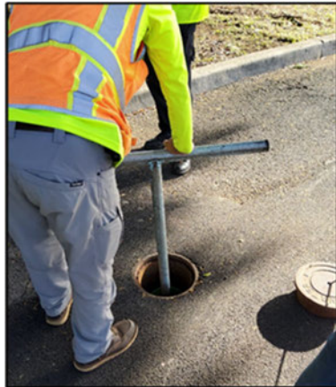
Figure 6-4 Valve Exercise with Valve Key
